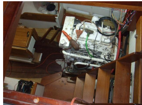
Engine room with small diesel
