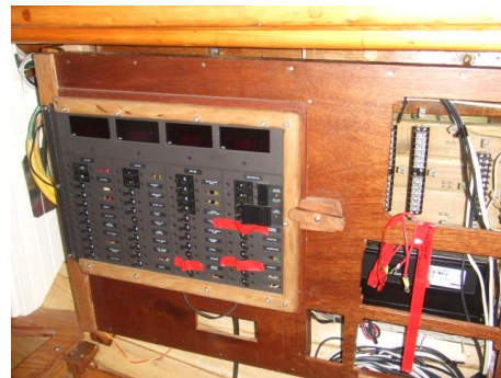
Instrument control panel
